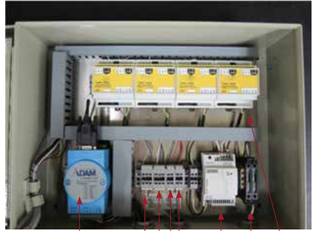
Figure 2: Interior of Enclosure
